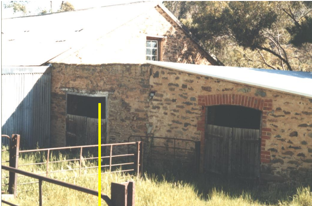
End of old shearing shed (with addition on right), Highland Valley (Photo: Wendy Baker 2002)
