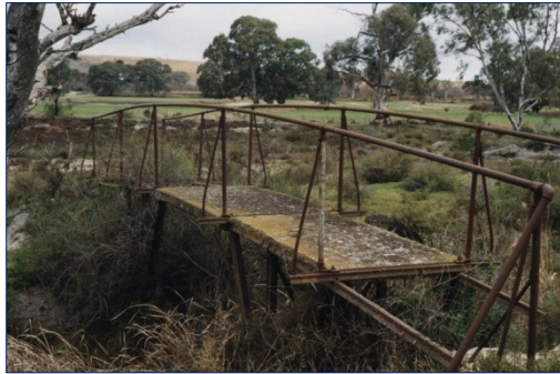
R.W. Clark's 89 year old prefabricated bridge at Mypolonga, as it was in 2003
